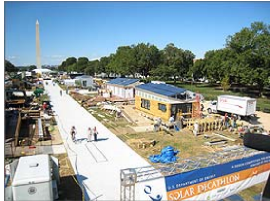
Construction is underway at the Solar Decathlon, which opens to the public on October 9. Enlarge this photo .
