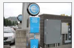
EV chargers at Lane Community College
